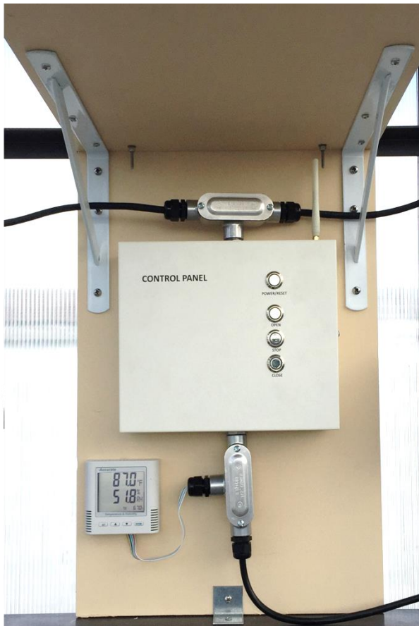
Typical wired control panel setup
