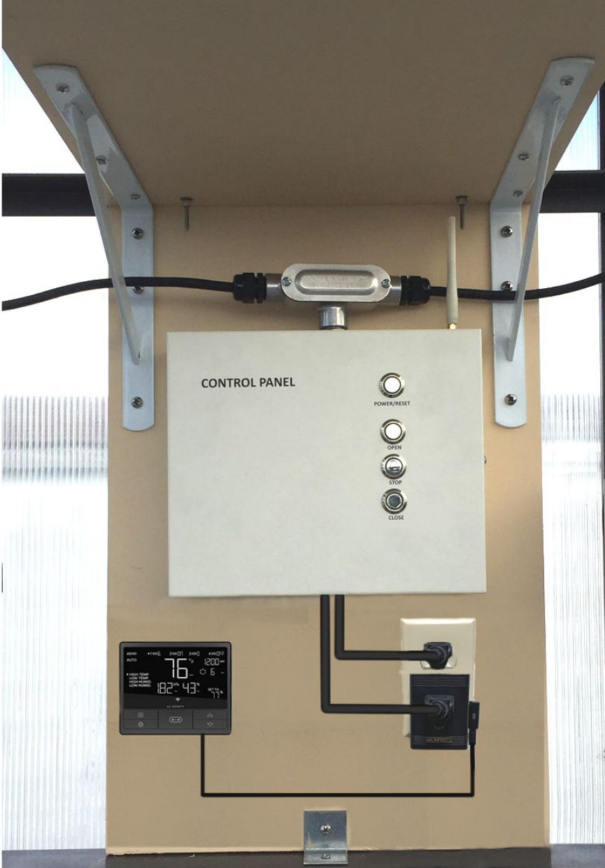
Typical control panel setup
